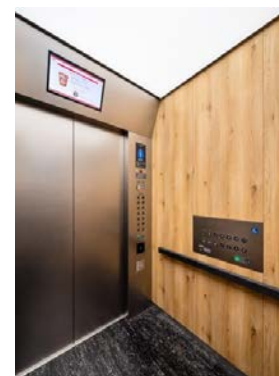
Nissin Foods Tokyo Head Office ( Tokyo, Japan ) 5 elevators
