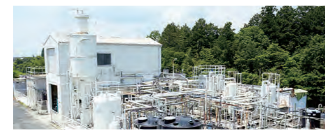
Wastewater treatment facilities at the Okayama Plant
