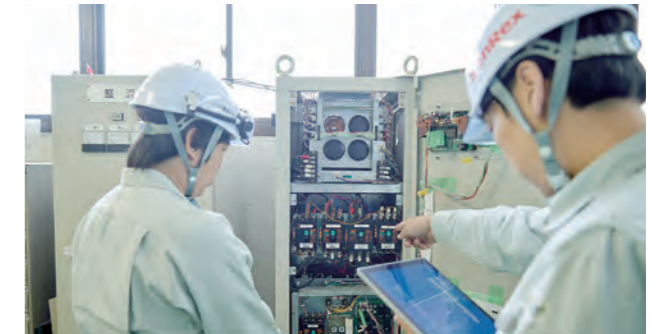
Power supply maintenance and inspection services
