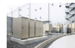
Emergency Power Supply
