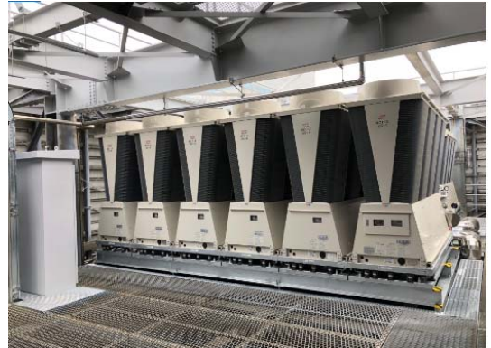
Installation of high-efficiency heat-source system(Shin-Yokoyama TECH Building)
