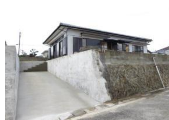
House where two parking spaces were created by removing garden trees and part of the retaining wall
