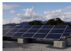
Hongo Photovoltaic Power Plant
