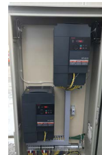
Inverter of a cooling water pump
