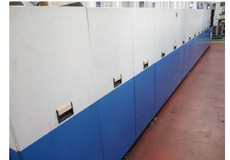
Heat treatment furnaces
