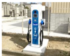
Electric vehicle charging station
