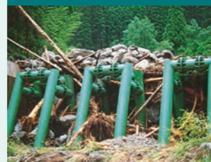
Capturing of giant rubble and driftwood in debris flow
