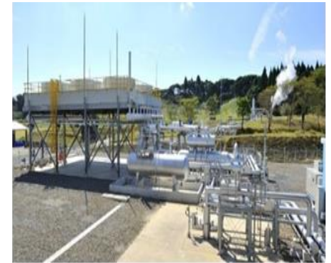
■ Geothermal power generation (Ibusuki City)
