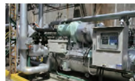
Fluorocarbon cooling equipment
