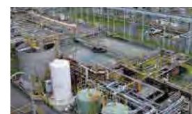
Activated sludge treatment facility
