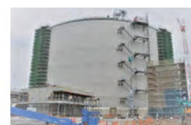
One of Japan's Largest LNG Tanks under Construction (At the Ehime Works Site)
