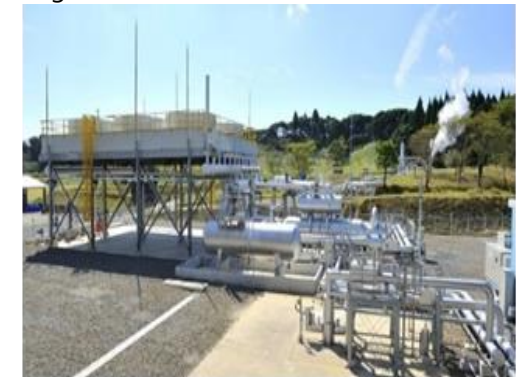
■ Geothermal power plant in Medipolis Ibusuki
