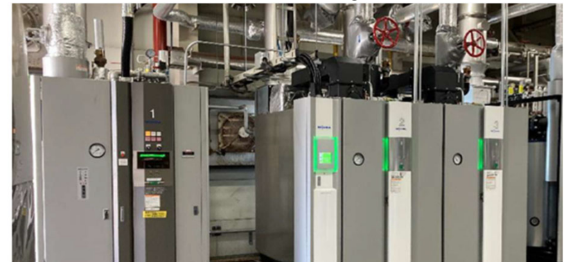
Introduced a boiler that can effectively use unnecessary oil as fuel in the factory (Kashima Oil Factory)
