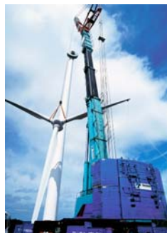
All terrain crane lifting the blades for assembly of an offshore wind turbine
