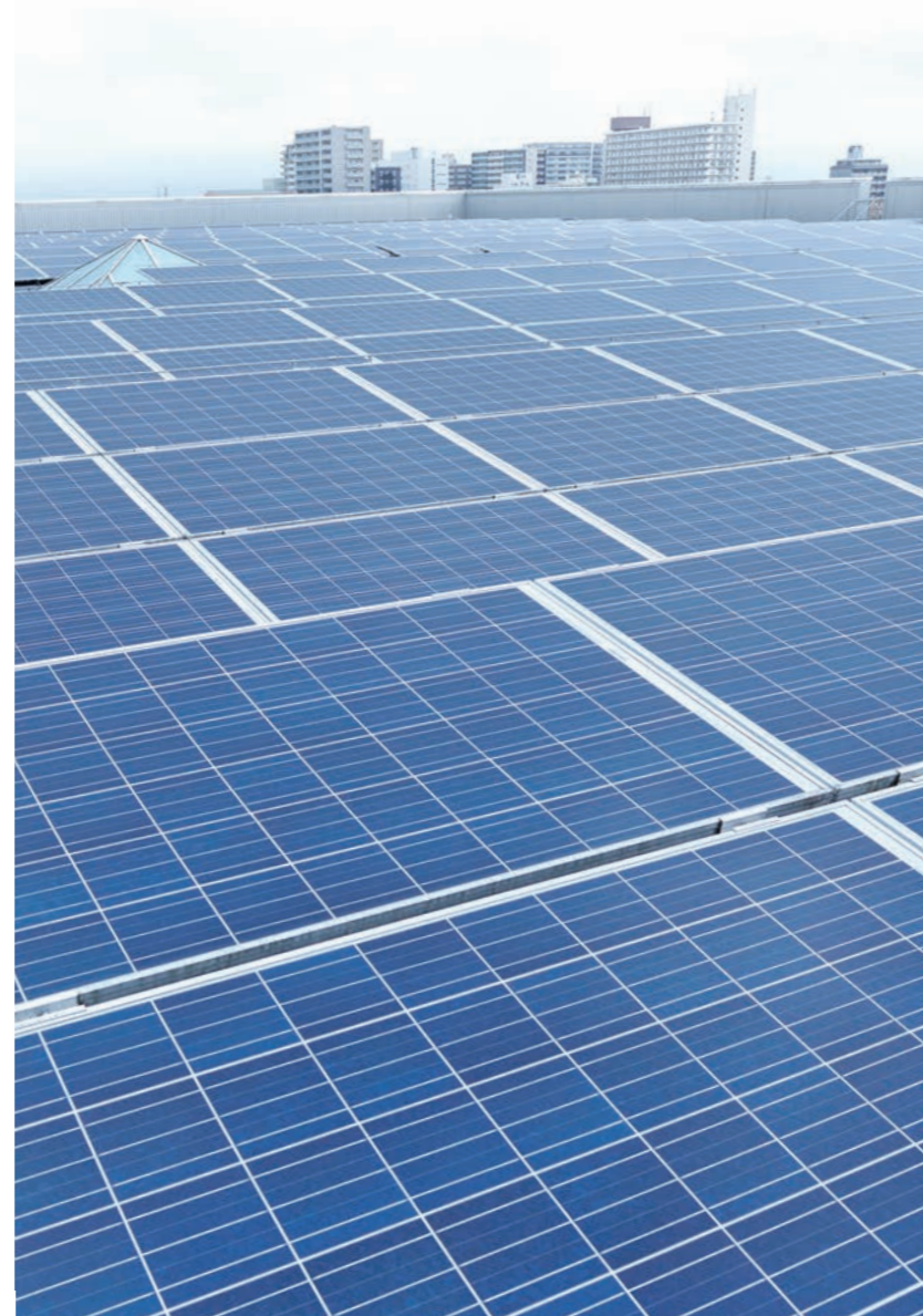
Solar panels installed on the roof of the Shiga Plant
