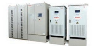
Power conditioner for the VPP demonstration installed in our former Osaka Plant
