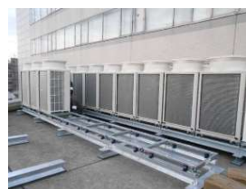
Renewal of air-conditioning system
