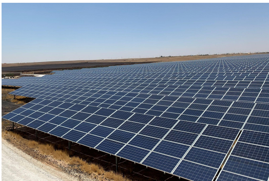
Solar power project with storage batteries in Al Badiya, Jordan
