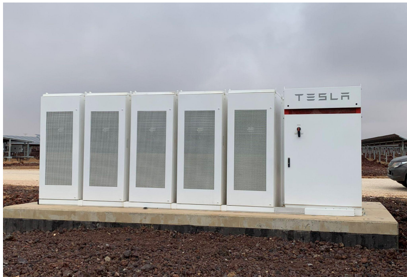
Tesla storage batteries installed in the site
