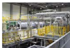
10MW-class alkaline water electrolysis plant
