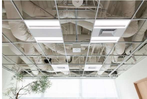
The office has been upgraded with additional construction to increase the ventilation performance so that the employees can feel safe.
