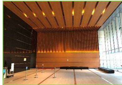
[Specific ceiling earthquake resistance measures] (NBF Toyosu Canal Front)
