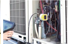
Pressure gauge connectivity
