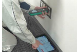
Electrical outlet testing
