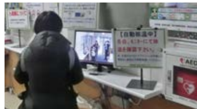
mozo wonder city Installation of temperature measurement equipment at all tenants' employee entrances
