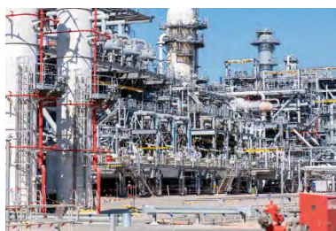
Onshore gas liquefaction plant
