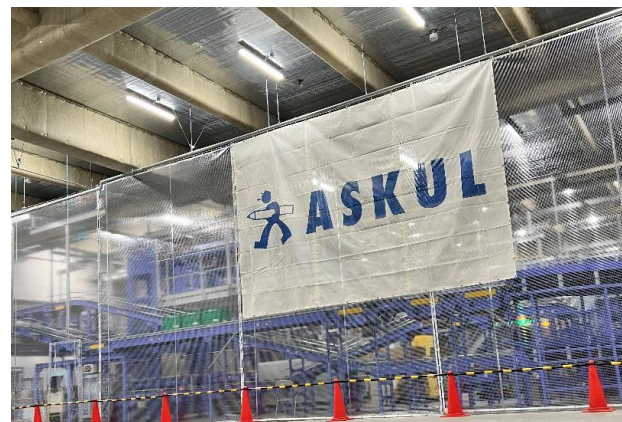
Conveyor transfer equipment
