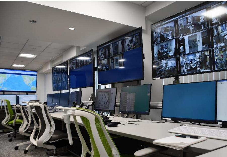
● CSC with enhanced equipment in Kanto Regional Office
