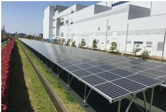
ROHM Hamamatsu's Solar Power System
