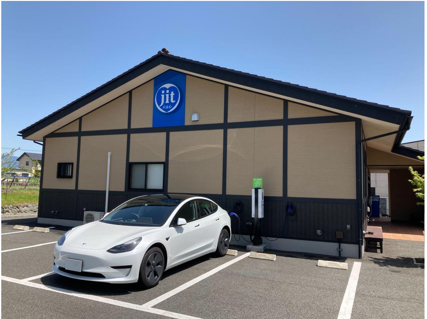
Charging station for ENECHANGE EV Charging Service installed at JIT Ceremony Wakakusa Hall
