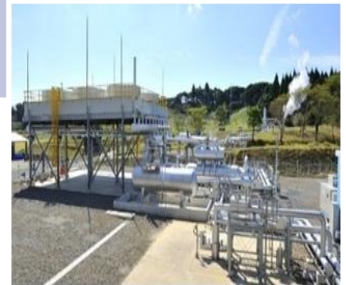
■ Geothermal power plant in Medipolis Ibusuki
