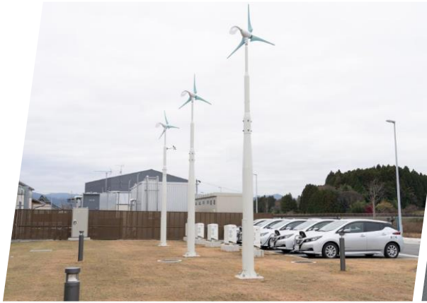
Energy management system
