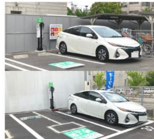
Osaka: Ecolocity Co., Ltd. (Parking lot at the prefectural government offices, 4 units)
