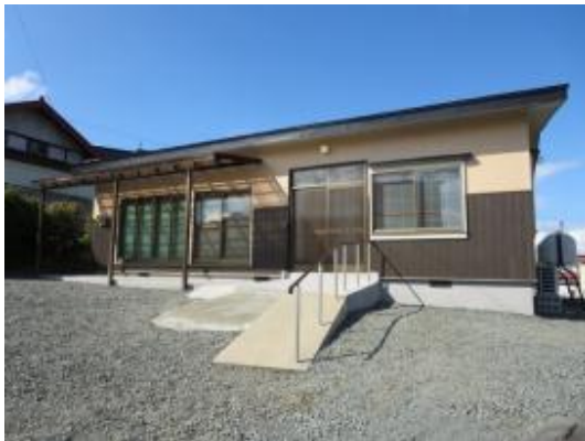
Renovated one-story house: replaced the damaged eaves and refreshed the dilapidated exterior
