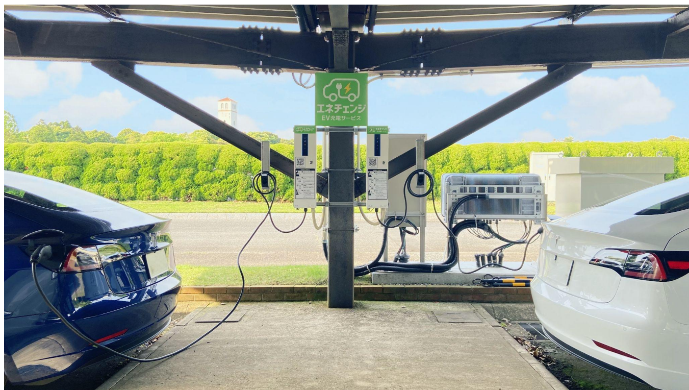
Charging station for ENECHANGE EV Charging Service installed at Yonehara Golf Club
