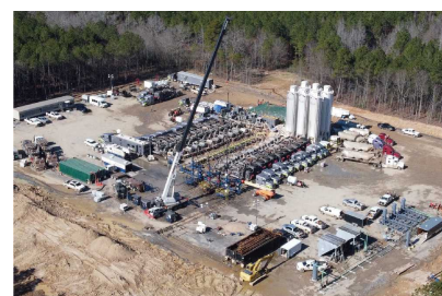
Shale gas mining area of Sabine Oil & Gas Corporation (Texas, US)
