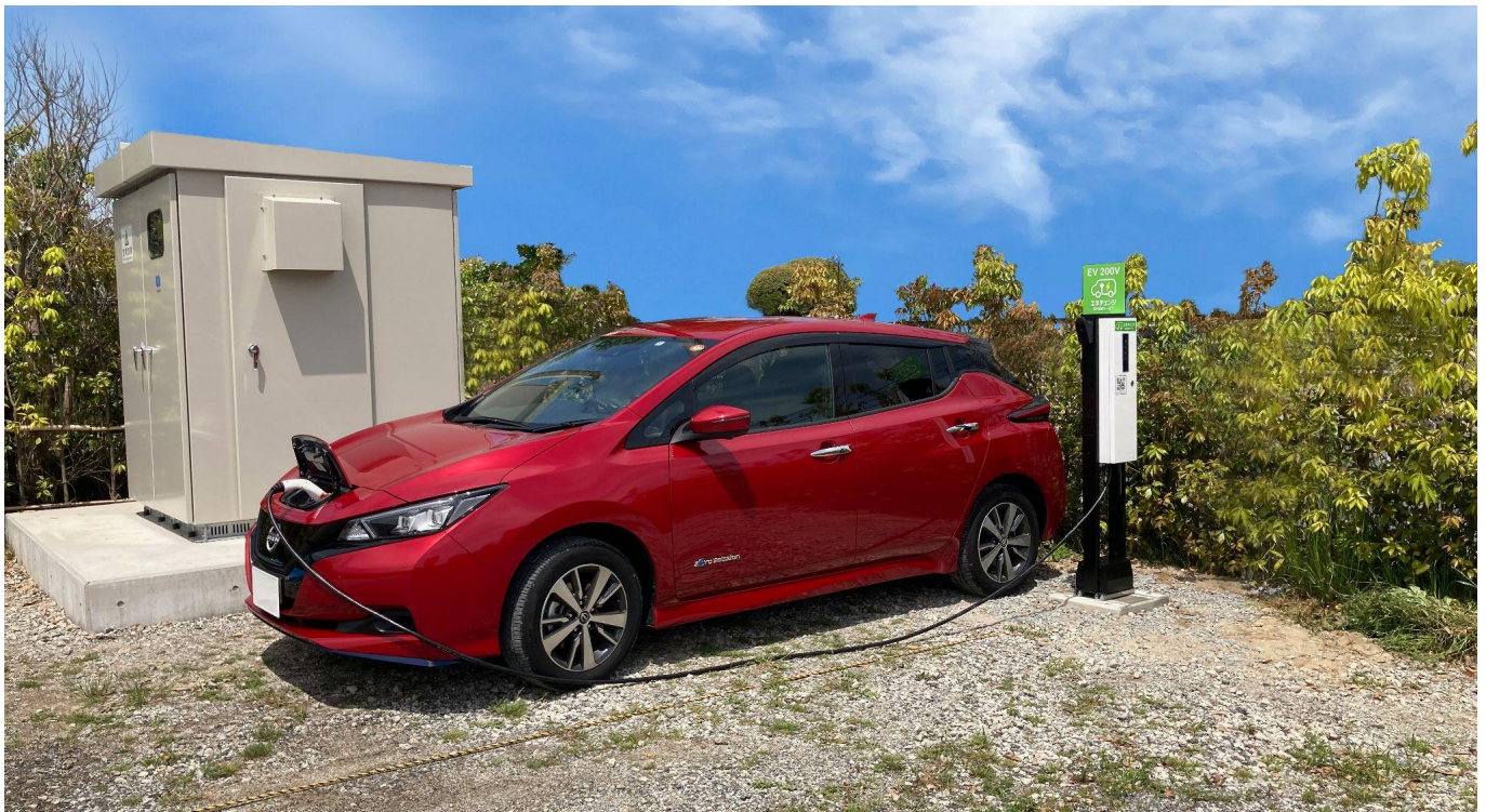
Charging station for ENECHANGE EV Charging Service installed at the Grand Dome Fukuoka Fukutsu
