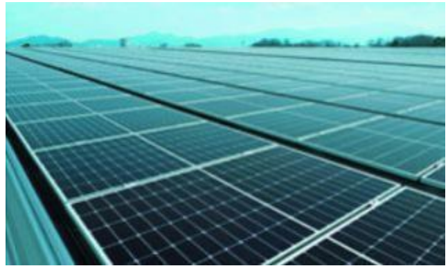
Photovoltaic power generation system
