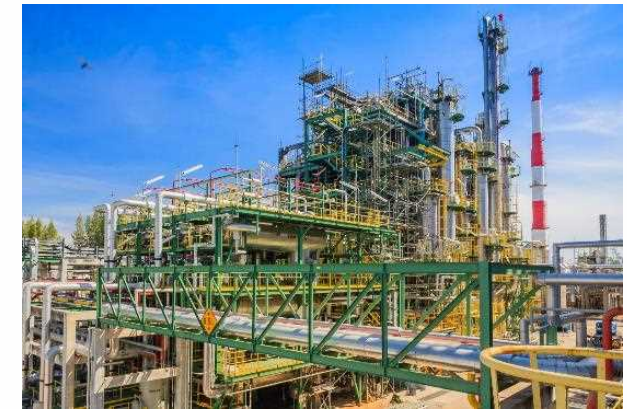
PCD plant in Thailand: Second manufacturing facility went into operation in October 2020, increasing production capacity to 8,000 tonnes per year.
