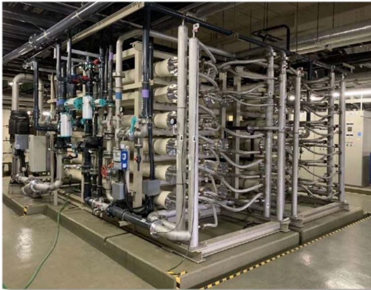
RO Membrane Facility
