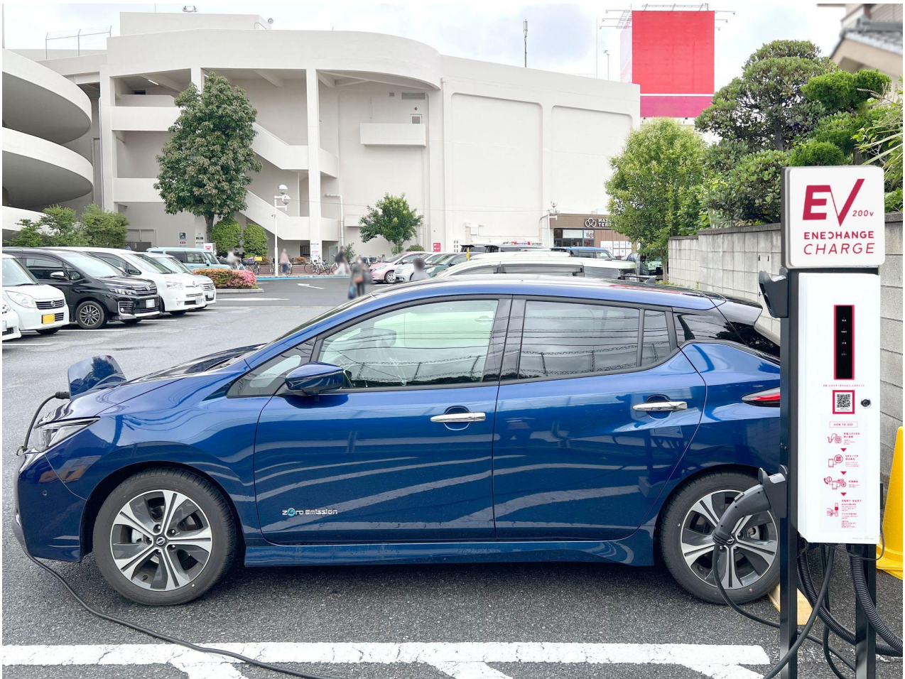
ENECHANGE EV Charging Service charging station installed at MATSUBARA TERRACE
