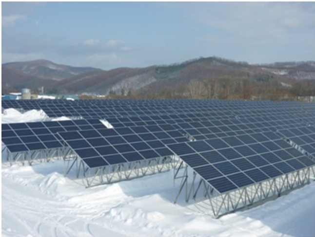
Ichigo Engaru Higashimachi ECO Power Plant (Hokkaido)
