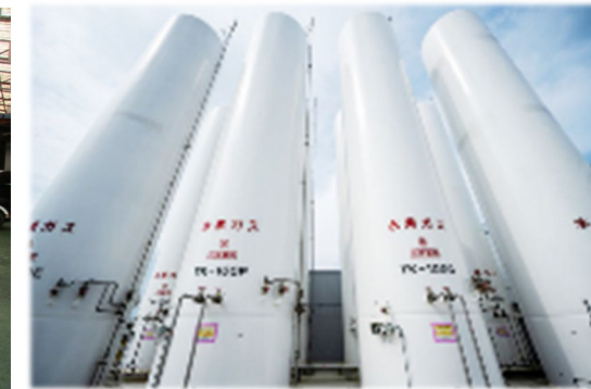
Hydrogen gas storage tank (manufactured by Fuji Car Manufacturing)
