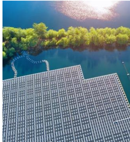
On-water solar power generation
