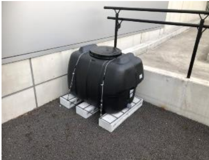
Install rainwater storage tanks to reuse rainwater for watering plants and exterior watering
