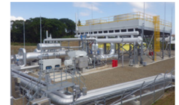
1,500kW-class geothermal power station
