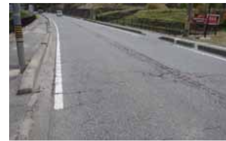
Damaged road pavement
