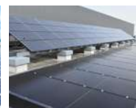
Solar power generation facility (Atsugi site)
