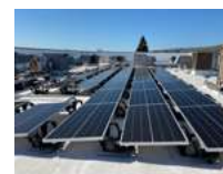
Solar power generation facility (U.S.A.)
