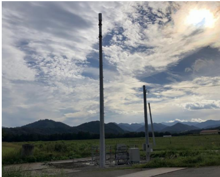
(Photo) Tower in Hiroo, Hokkaido (Before the installation of base stations)
