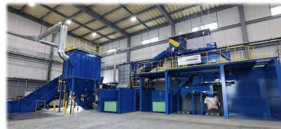
Crushing line for electronic waste
