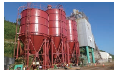
Dedicated "ash-crete" plant.
