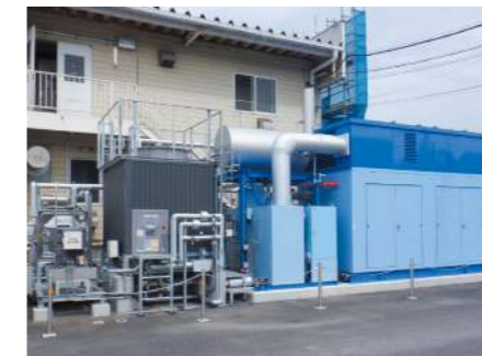
Cogeneration system deployed at the Asakusa Ham's Kanto Plant
