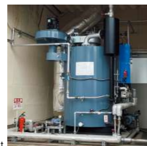
Cooking oil waste boiler used in the Tohoku Plant
