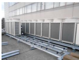
Renewal of air-conditioning system
