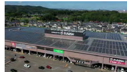
Solar power system installed at the Home Center Musashi store in Natori
