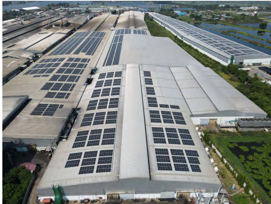
Solar power systems installed on the roofs of the plant
